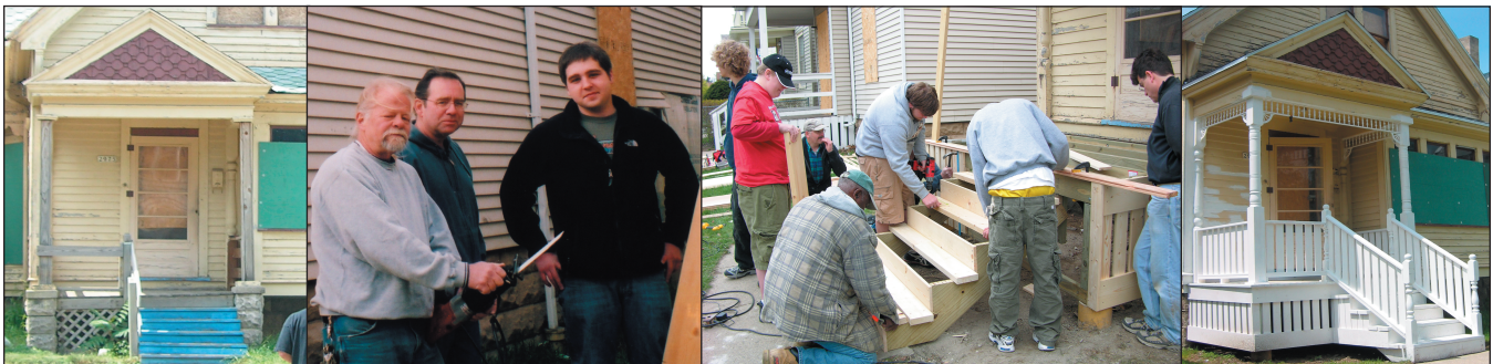
Tyler Holst, seen in the red shirt above, restored the delapidated porch at 2975 North 21 st Street for his final Eagle Scout Project. The porch was completed along with his troupe and father Jim Holst, seen above brandishing a sawzall with others from the Boy Scouts.
