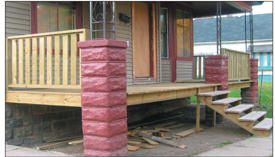
Nicole Lestor's porch is nearly completed after the volunteer crew finishes their work.
